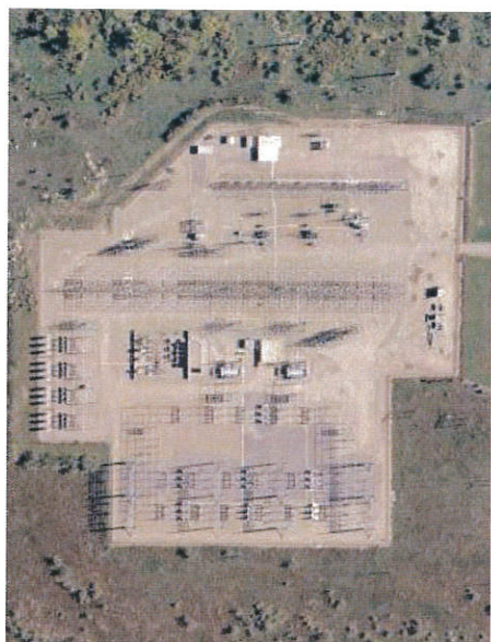
Above: Camp Williams Substation. 345 kV to 138 kV, 138 kV to 12.5 kV. Below: 90th South Substation 345 kV to 138 kV, 138 kV to 46 kV, 138 kV to 12.5 kV.
