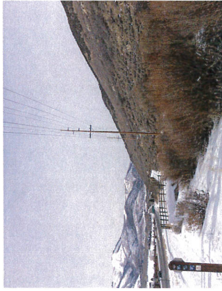
Transmission line co-located with a trail near HWY 224 in Snyderville Bosnia
