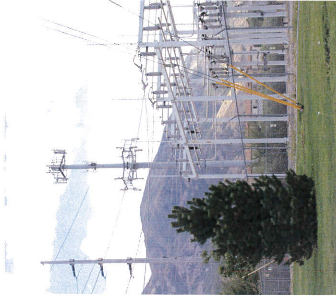
Co-location of telecommunication towers with substations
