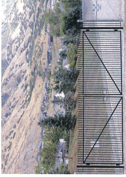
Berms and slopes are used to integrate a substation into the surrounding neighborhood
