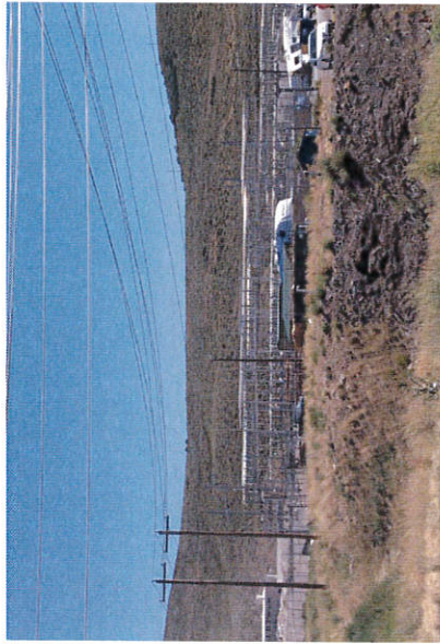
Above: Southeast Substation Regional with Distribution. 138 kV to 12.5 kV Below: Silver Creek Substation 138 kV to 46 kV, 138 kV to 12.5 kV.
