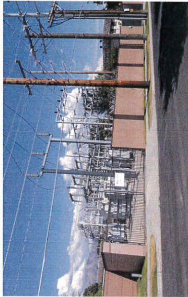
Above: Meadowbrook Substation aerial view. Below: Meadowbrook Substation street view. 138 kV to 12.5 kV.
